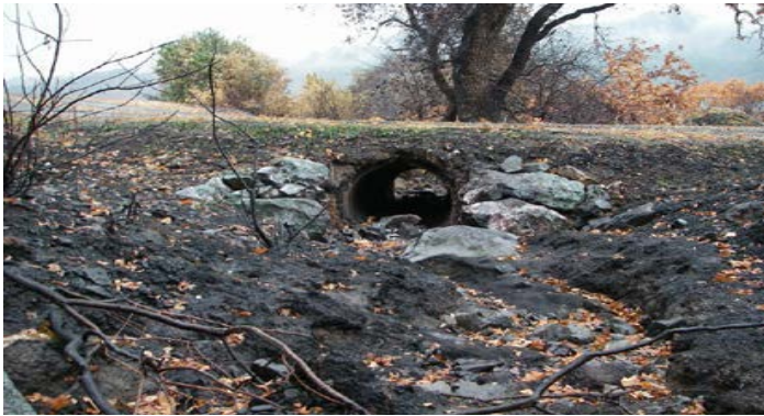
Burned Out Culvert at Site 4. Photo by Pacific Watershed Associates.
